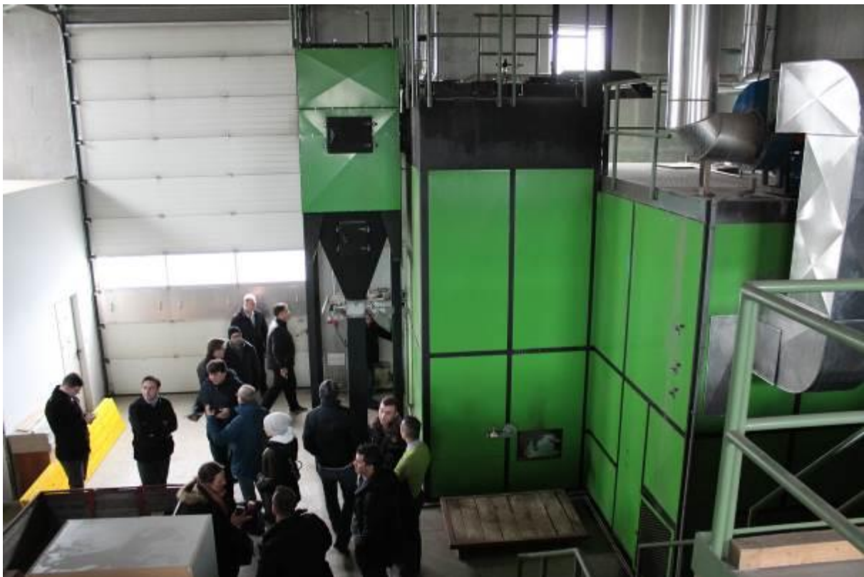
Figure 11: Biomass boiler with 1,700 kW
