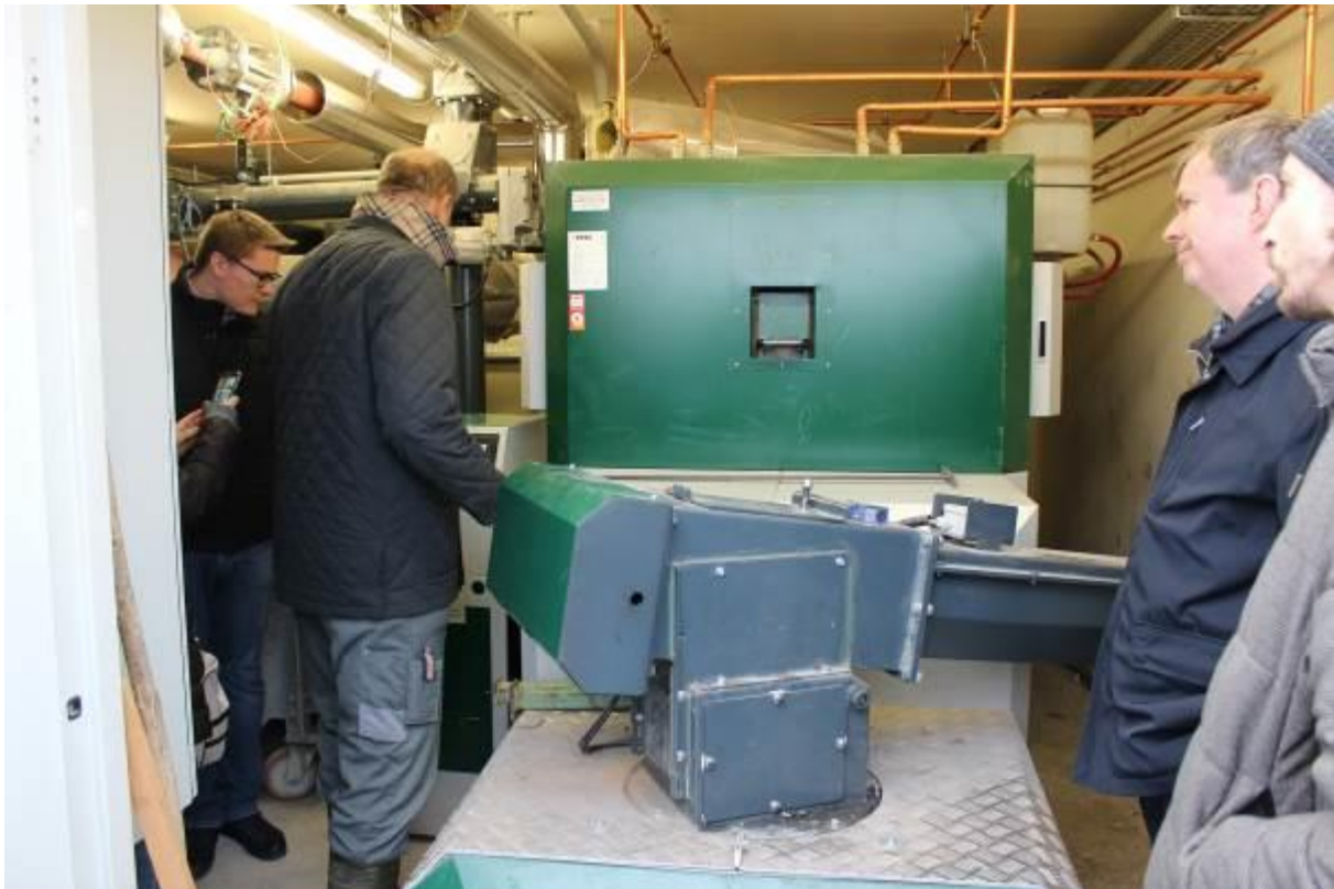
Figure 6: Biomass boiler with about 390 kW thermal capacity
