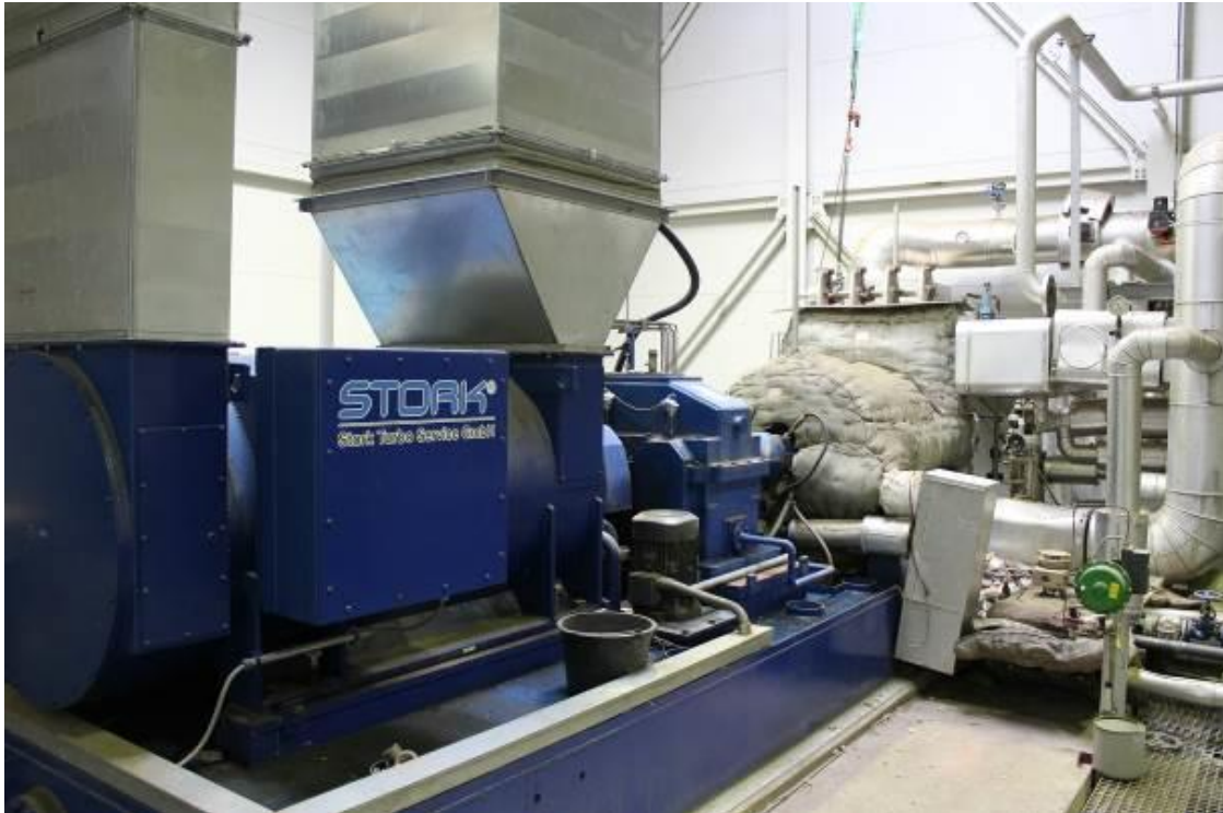
Figure 17: Steam turbine and generator
