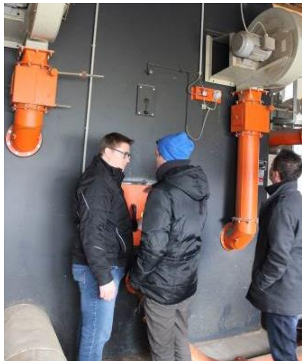
Figure 16: Boiler operated with saw dust as a fuel
