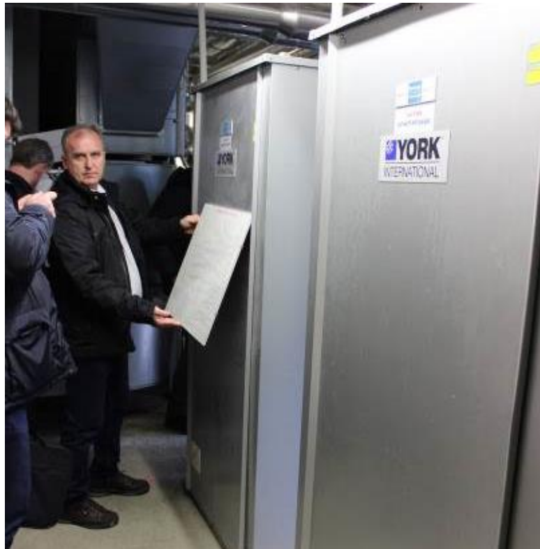
Figure 13: Absorption chillers at the centre of technologies in Güssing
