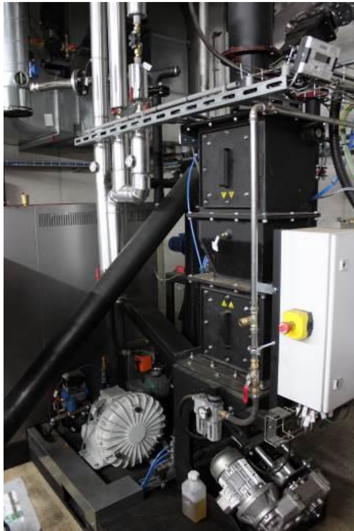
Figure 3: Gasifier unit of the CHP
