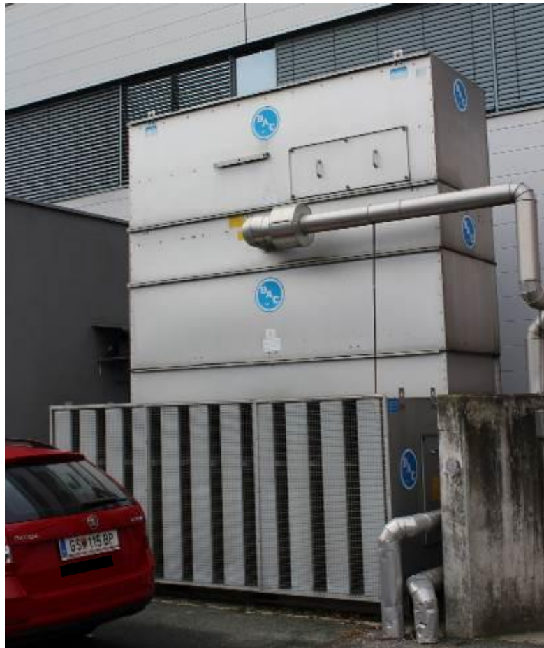
Figure 14: Wet cooling tower for the absorption chiller
