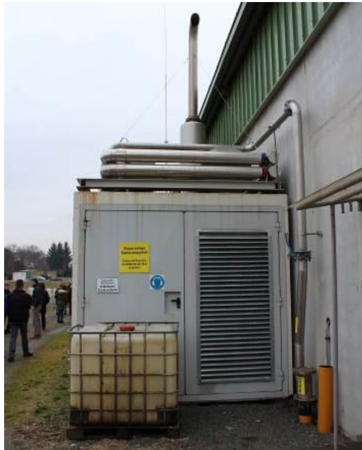
Figure 12: Biogas engine for the DH grid
