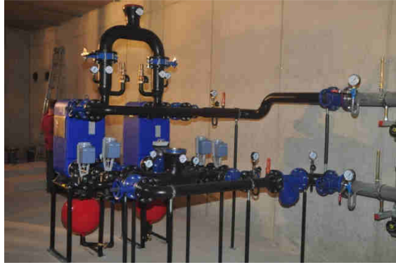
3,5MW station for MedCampus in Graz
